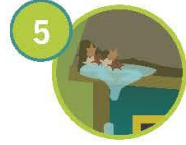
5 Clogged rain gutter (home and street)
